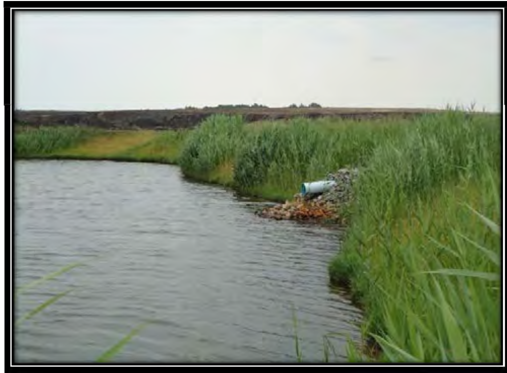
Photo 21 – Discharge Pipe from Ash Pond 2 into Pond 4
