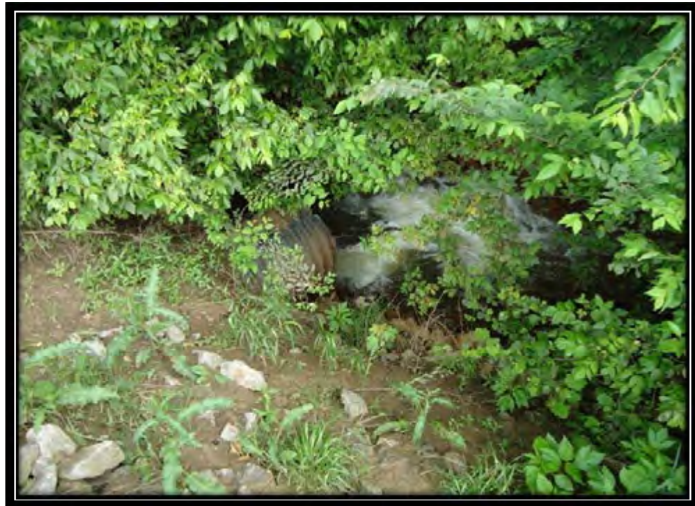
Photo 28 – Corrugated Metal Pipe Outfall from Ash Ponds to the South Fork of Little Saline Creek May 25, 2011 IL50160
