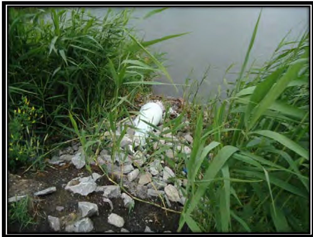
Photo 20 – Discharge Pipe from Ash Pond 1 into Pond 4
