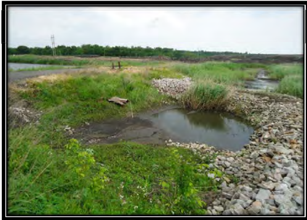
Photo 13 – Ash Pond 2 Discharge Pipe into Ash Pond 4 May 25, 2011 IL50160
