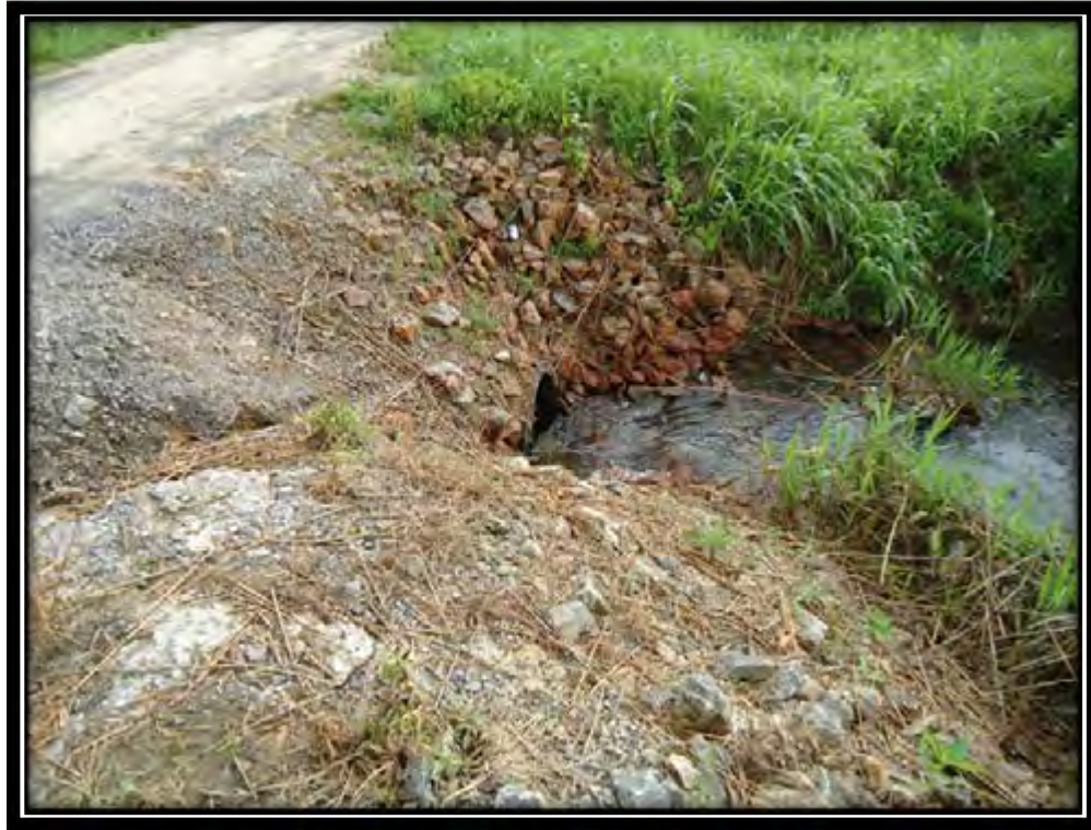
Photo 27 – Corrugated Metal Pipe under Access Road Leading to Outfall Downstream of Pond 4 May 25, 2011 IL50160
